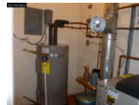
Hot Water Heater
