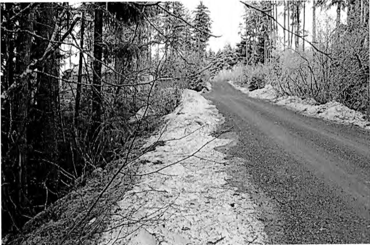
Side of Shared Driveway showing drop-off.JPG
