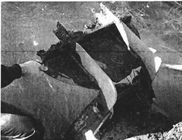
Figure 11. West berm failed culvert flap.
